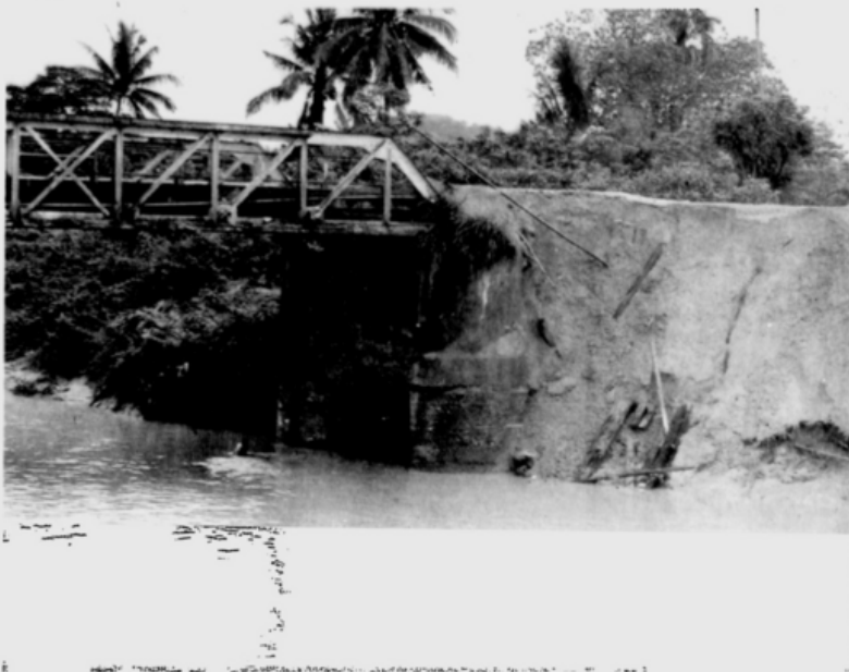
Danger of collapse...a slice of the river embankment by the old steel bridge in the former West Country Estate has been eroded away.
