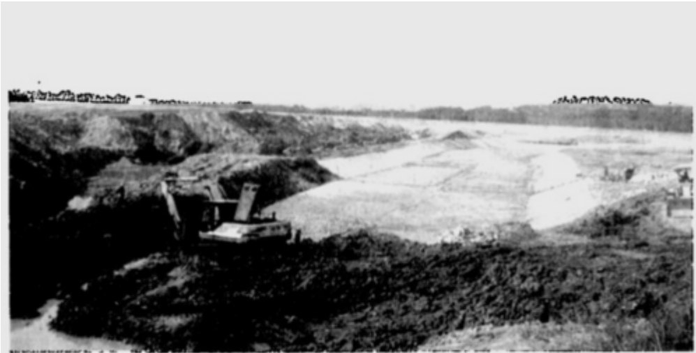
WORK IN PROGRESS ... to level the river bed of Sungai Air Hitam and developed it into a lake garden.
