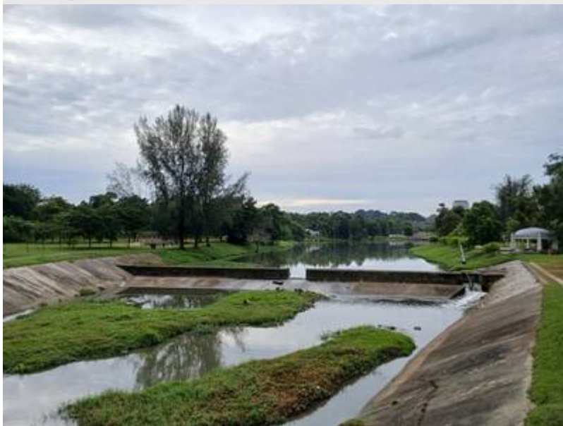
Kiri: Tasik yang hampir siap dibina. Gambar mungkin diambil di jambatan Sungai Air Hitam, Persiaran Bangi, menghadap ke selatan: “Work in progress ... to level the river bed of Sungai Air Hitam and developed it into a lake garden.”
