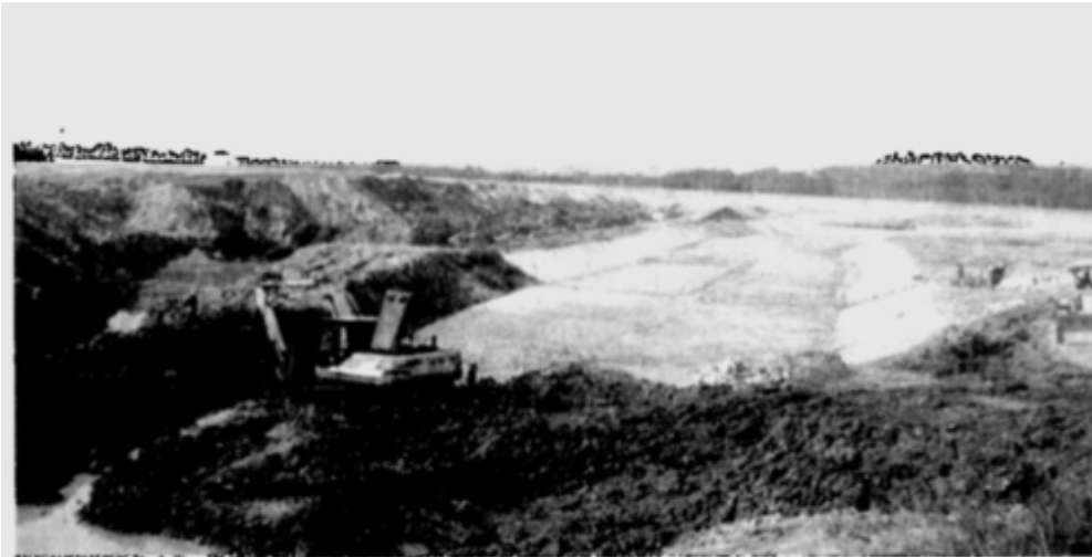
WORK IN PROGRESS ... to level the river bed of Sungai Air Hitam and developed it into a lake garden.
