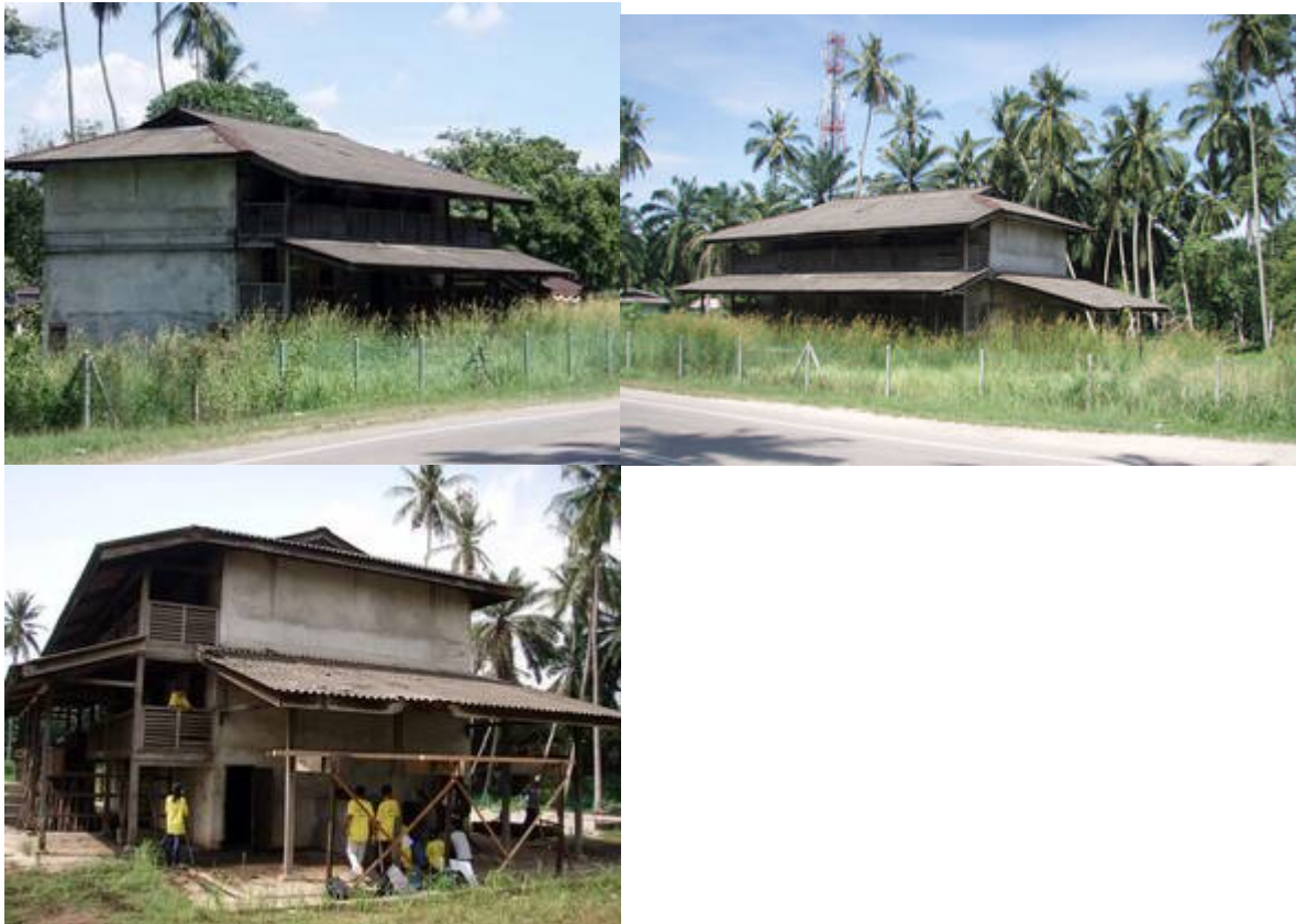
Sebelum dibaikpulih. Kiri: “Blackened, abandoned, dilapidated and ignored (2006)” . Tengah: “The rubber smokehouse before restoration” . Kanan: “Children learning how to conduct a dilapidation survey (2006)”
