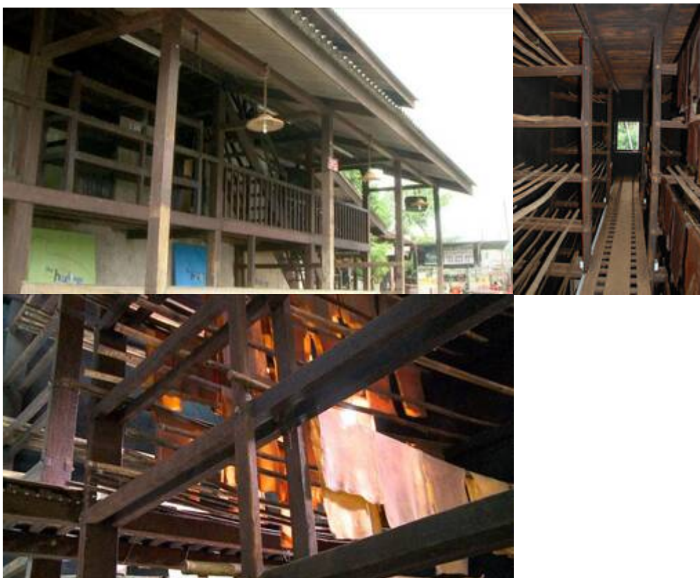
Setelah dibaikpulih. Kiri: “Racks of smoking room for rubber sheets hung on bamboo poles (2007)” . Tengah: “Racks of smoking room for rubber sheets hung on bamboo poles (2007)” . Kanan: “The timber in the Smokehouse was found intact and well preserved. Years of smoking the rubber, and by association the timber, had not only preserved the wood but also hardened it further (2010)” .
