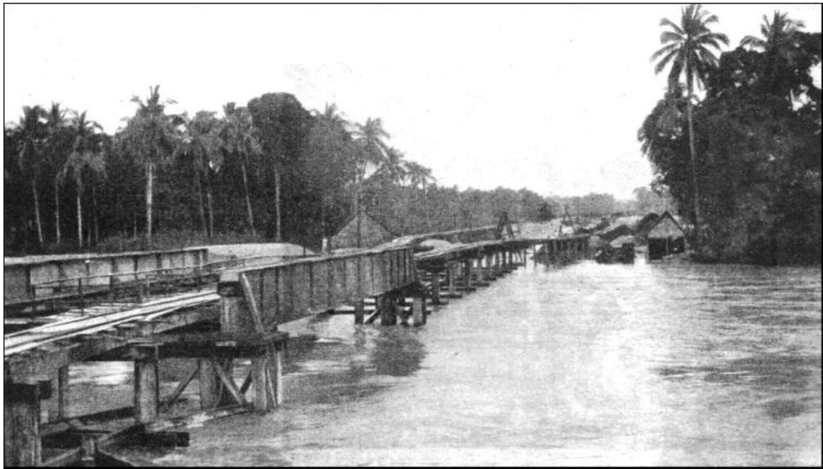
ENDANGERING THE WORK IN PROGRESS. The Muda River in Kedah overflowing its banks, threatening a bridge-building site.
